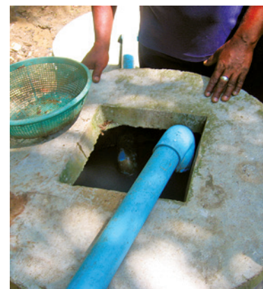
Close up of water treatment facility, Phuket, Thailand © S. Sereepaowong
