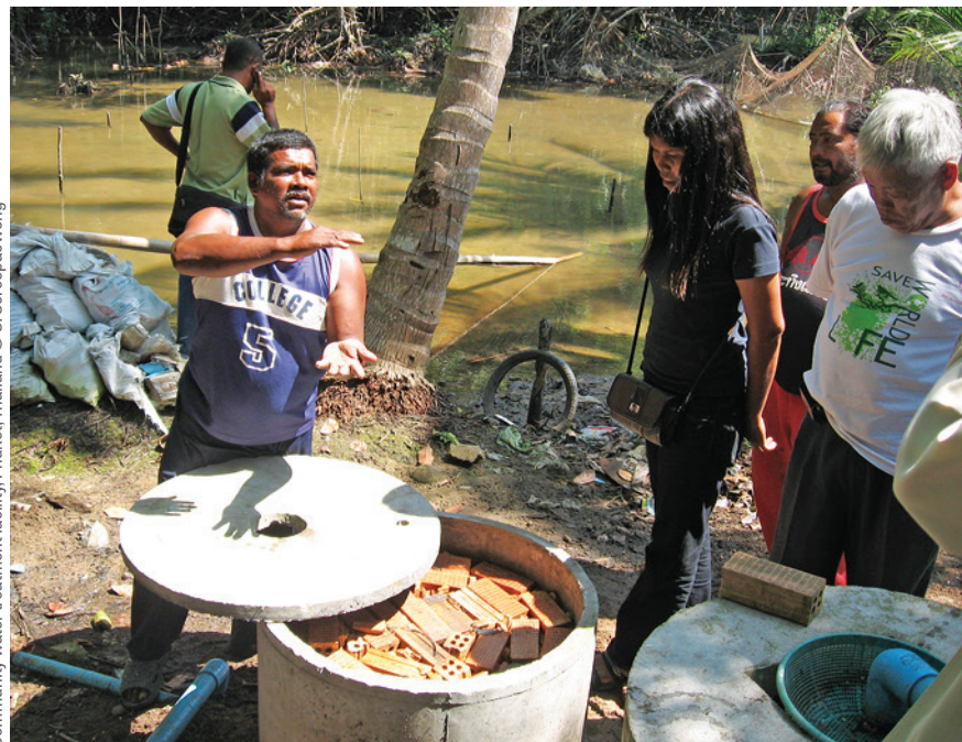
Community water treatment facility, Phuket, Thailand © S. Sereepaowong
